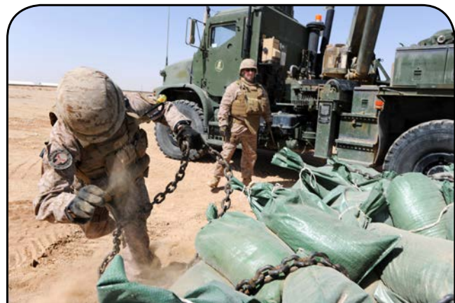
Builder 3rd Class Joseph Flowers, assigned to the Naval Mobile Construction Battalion (NMCB) 15's Convoy Security Element, throws chains under a pallet of sandbags while constructing a bunker in support of the Afghanistan National Army. (U.S. Navy photo by Mass Communication Specialist 2nd Class Daniel Garas/Released)
