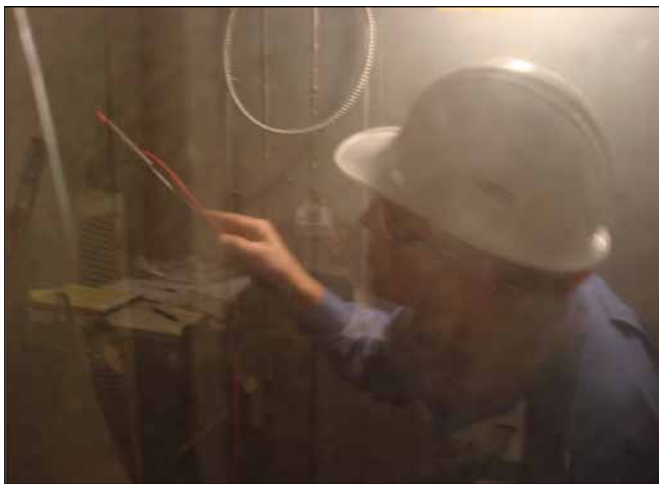
Figure 6—Unlike Motor #1, the Motor #2 shaft is difficult to reach, with only a couple of inches between the end-bell and a sheave exposed; the versatility of the splitting Aegis SGR and ease of installation using conductive epoxy become even more apparent.
