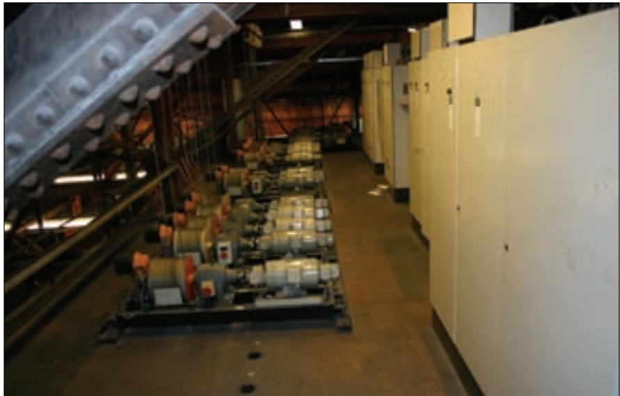
A total of 39 Sprint Electric DC drives were installed to extend the lives of the theatre’s existing motors (courtesy of Sprint Electric).
