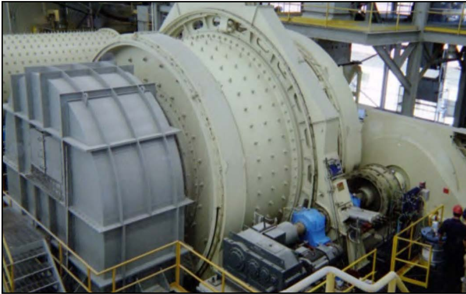
Figure 2 Grinding mill installation.
