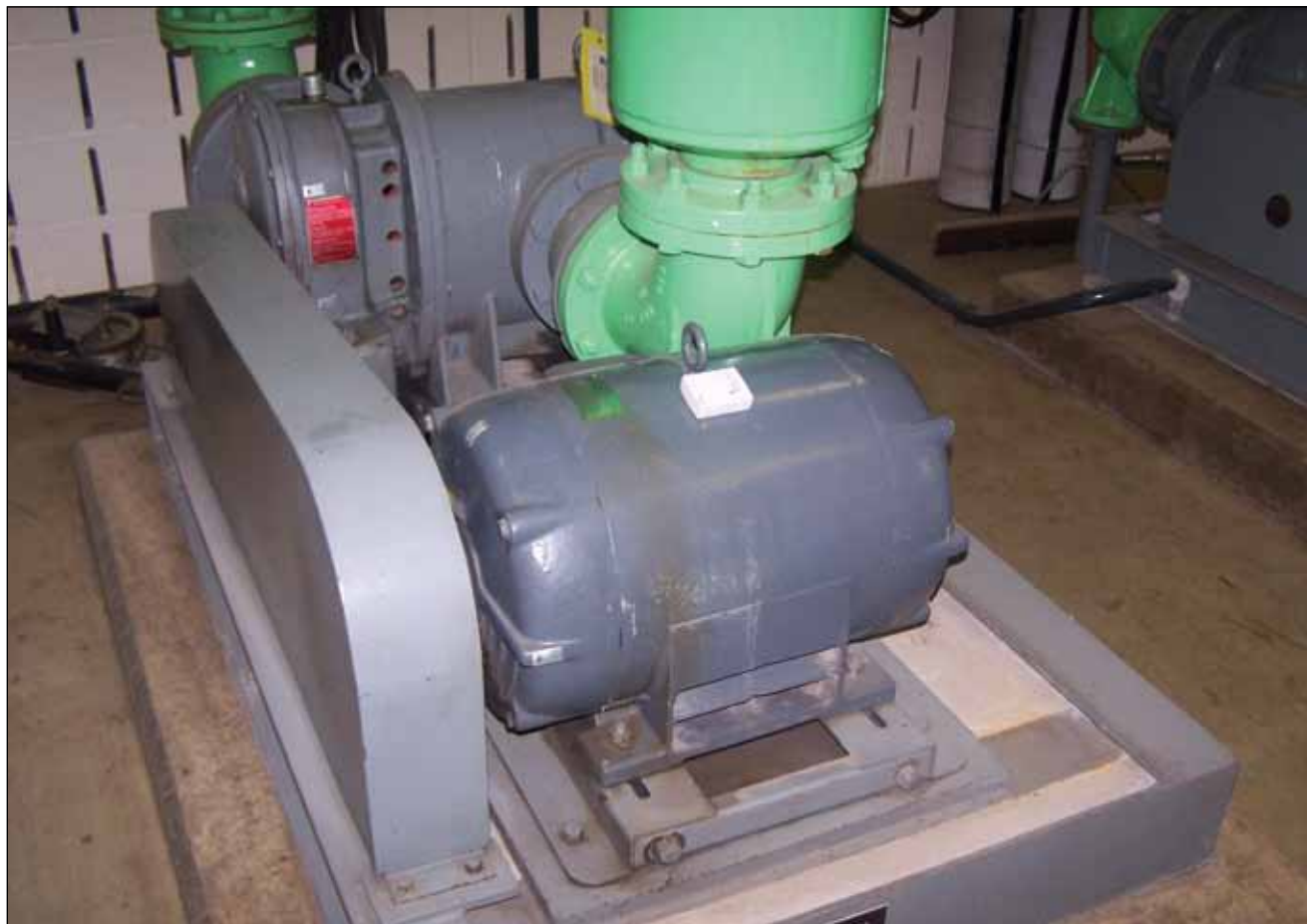
The data loggers were deployed on the motors (as pictured above), although some of the casings were too large to produce a good field reading, so they were also tied to feeders in the electrical cabinets.
