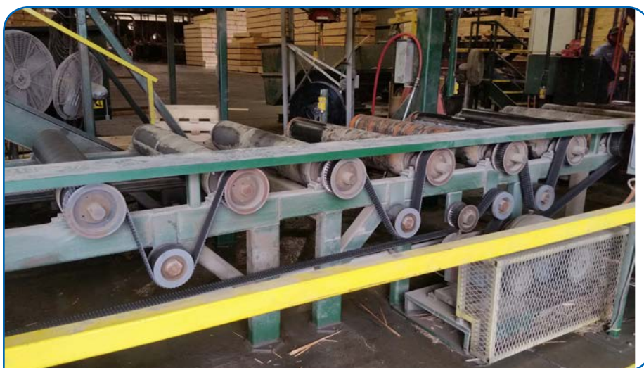
Figure 1 A lumber mill roll case requiring careful synchronization and smooth operation for stacking of boards got what it needed from Gates Corp.'s poly chain GT carbon extended length belt (courtesy Gates Corp.).
