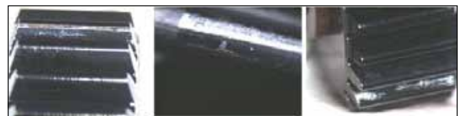
Figure 19—Coating damage after vibration.
