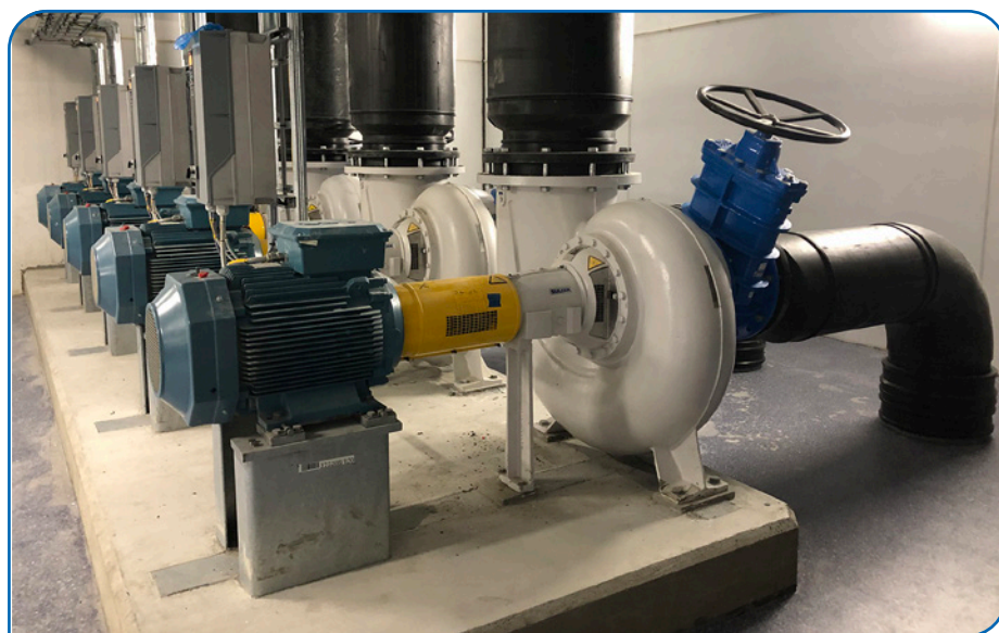
Five AHLSTAR A43-500 recirculation pumping units for brackish water.
