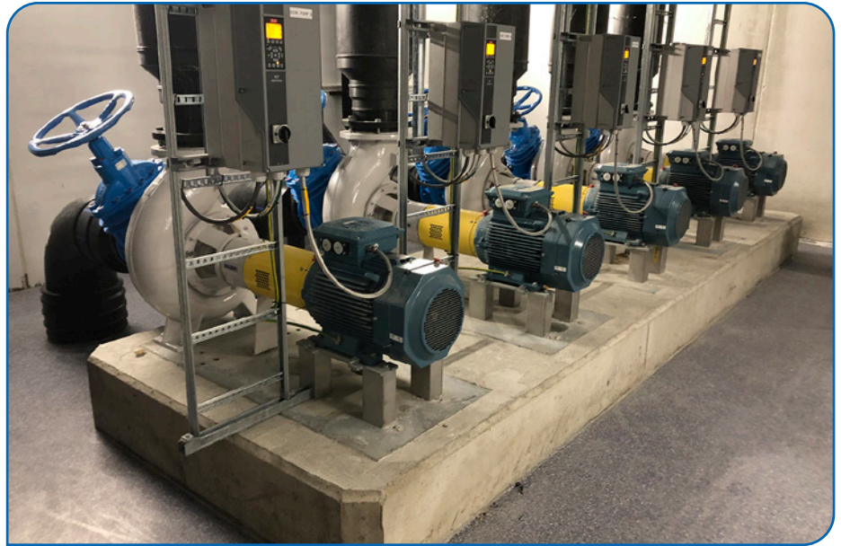
Five BE325-2532 recirculation pumps offer a huge energy savings and smaller total cost of ownership.
