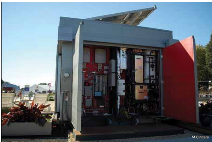
All of Lumenhaus’s components and systems are designed and built to work together to maximize user comfort with environmental protection. At its heart is an integrated, environmental control system (courtesy M. Cincala).
