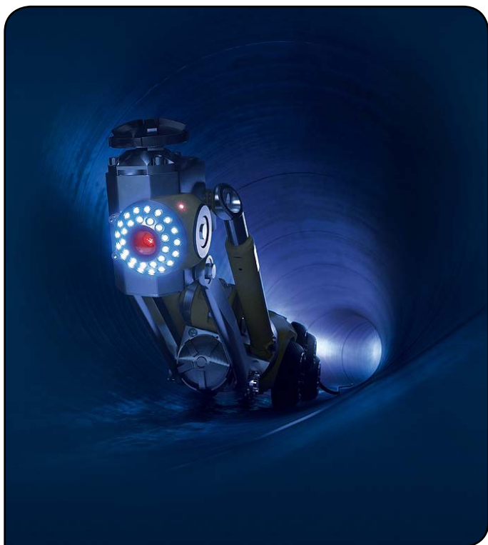
Figure 1 In the past, it was necessary to expose underground pipelines over long stretches just to localize damage. Today, sewer robots perform the assessment with no construction work at all (courtesy of Regelmann).
