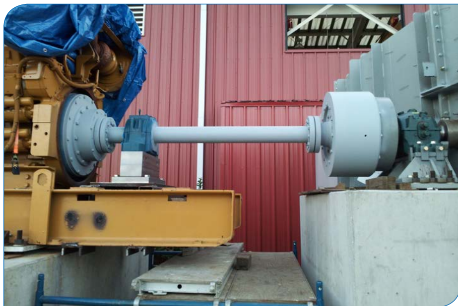
Engine/Blower drivetrain features left to right, engine, coupling, bearing assembly, shaft drive ring, Wichita clutch, bearing assembly and blower assembly.
