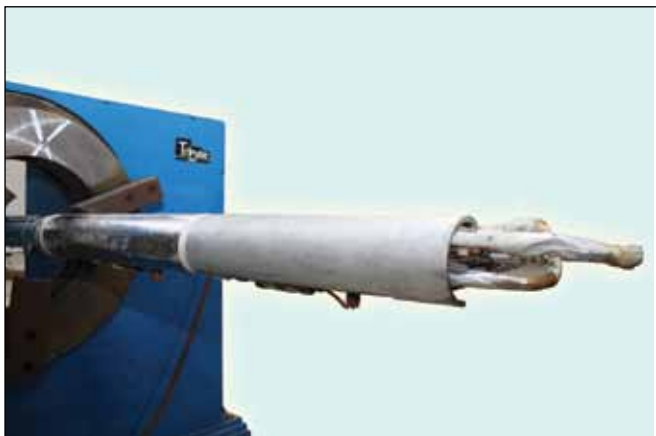
The dual-torch oscillation process involves feeding corrosion-resistant alloy wire into a 20-foot long torch that welds it along the inner wall of the steel pipe.
