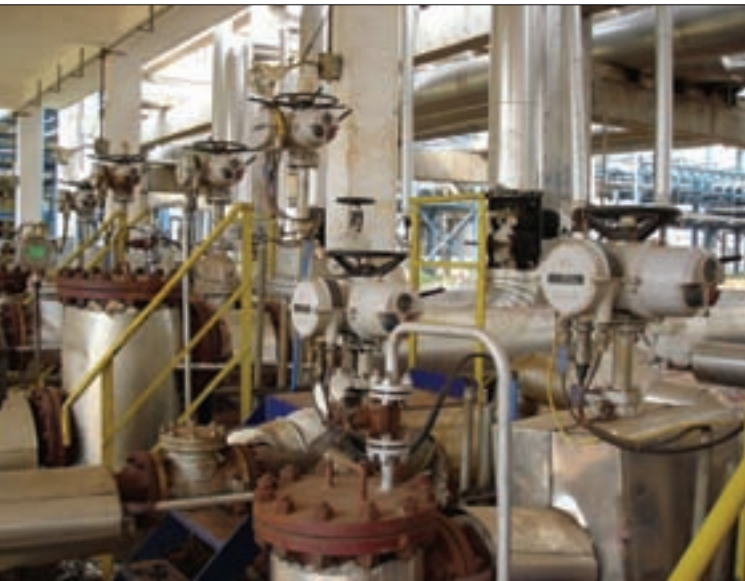
Rotork IQPro valve actuators were installed in a processing area of the Qinzhou Refinery.
