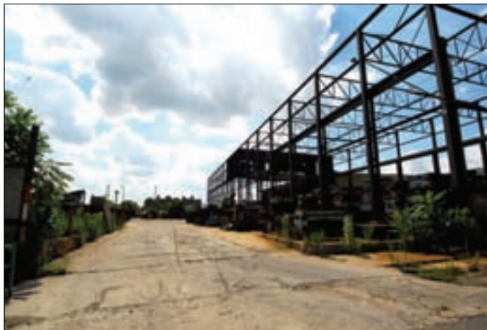
Construction on 23rd Street Studios will include LEED practices that focus on green manufacturing initiatives (Courtesy 23rd Street Studios).
