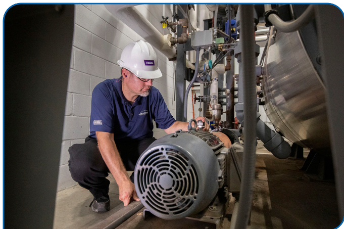
Perceptive Technologies install.
