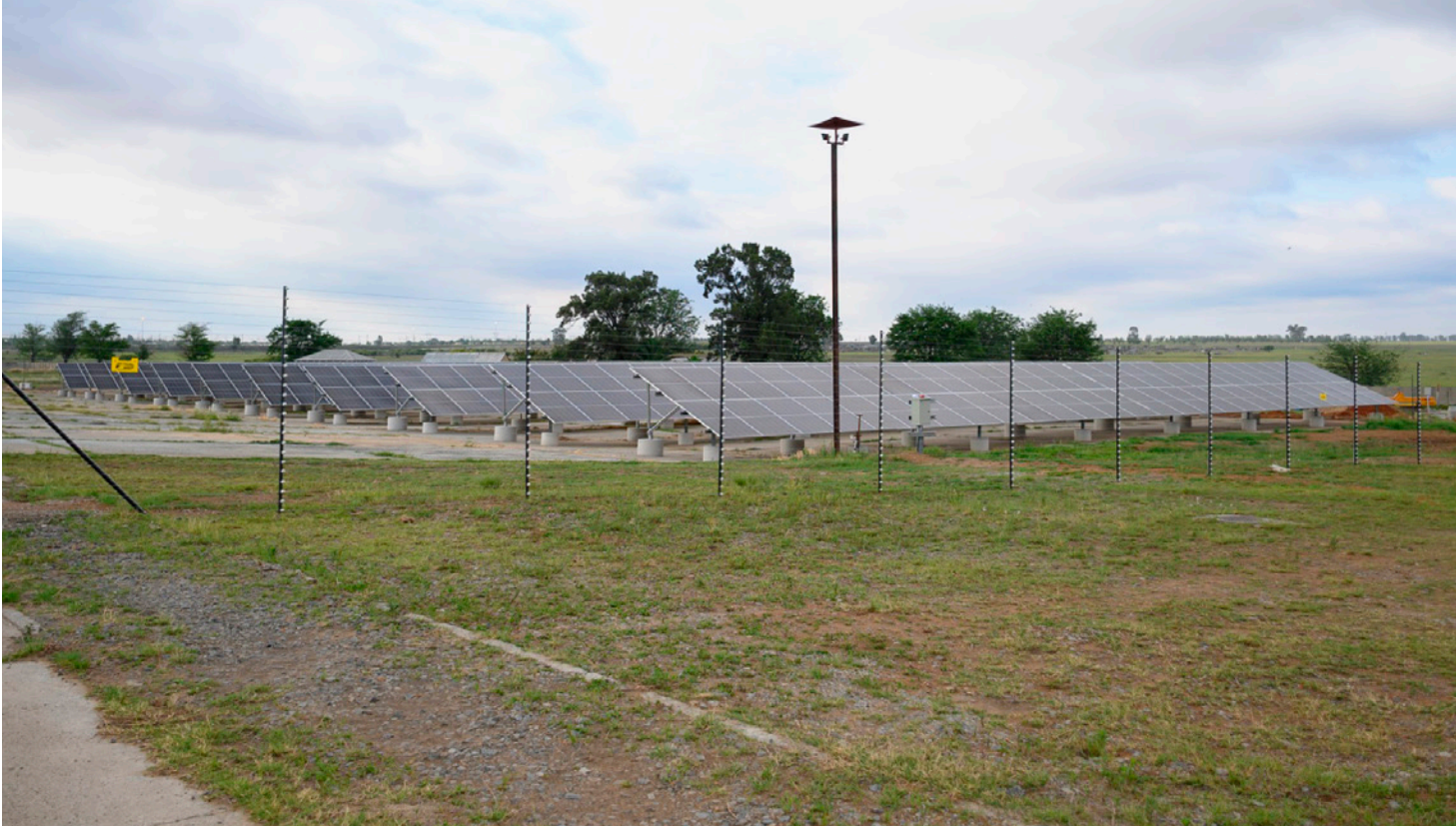
On-site at Vesconite Bearings, where the company is installing a comprehensive solar energy solution.
