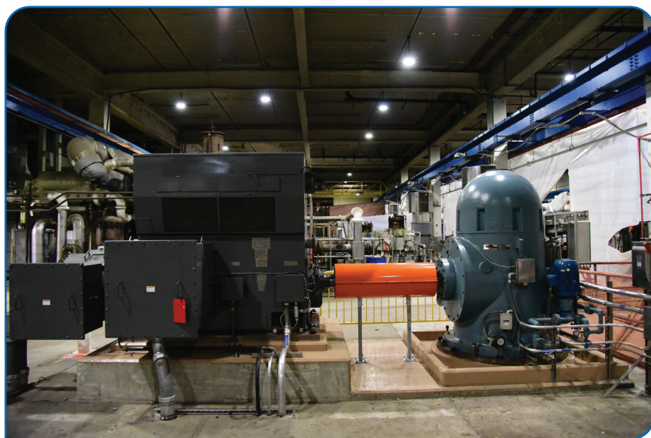
Philadelphia Gear drivetrain system includes new electric motor, right-angle pump drive, and control system.
