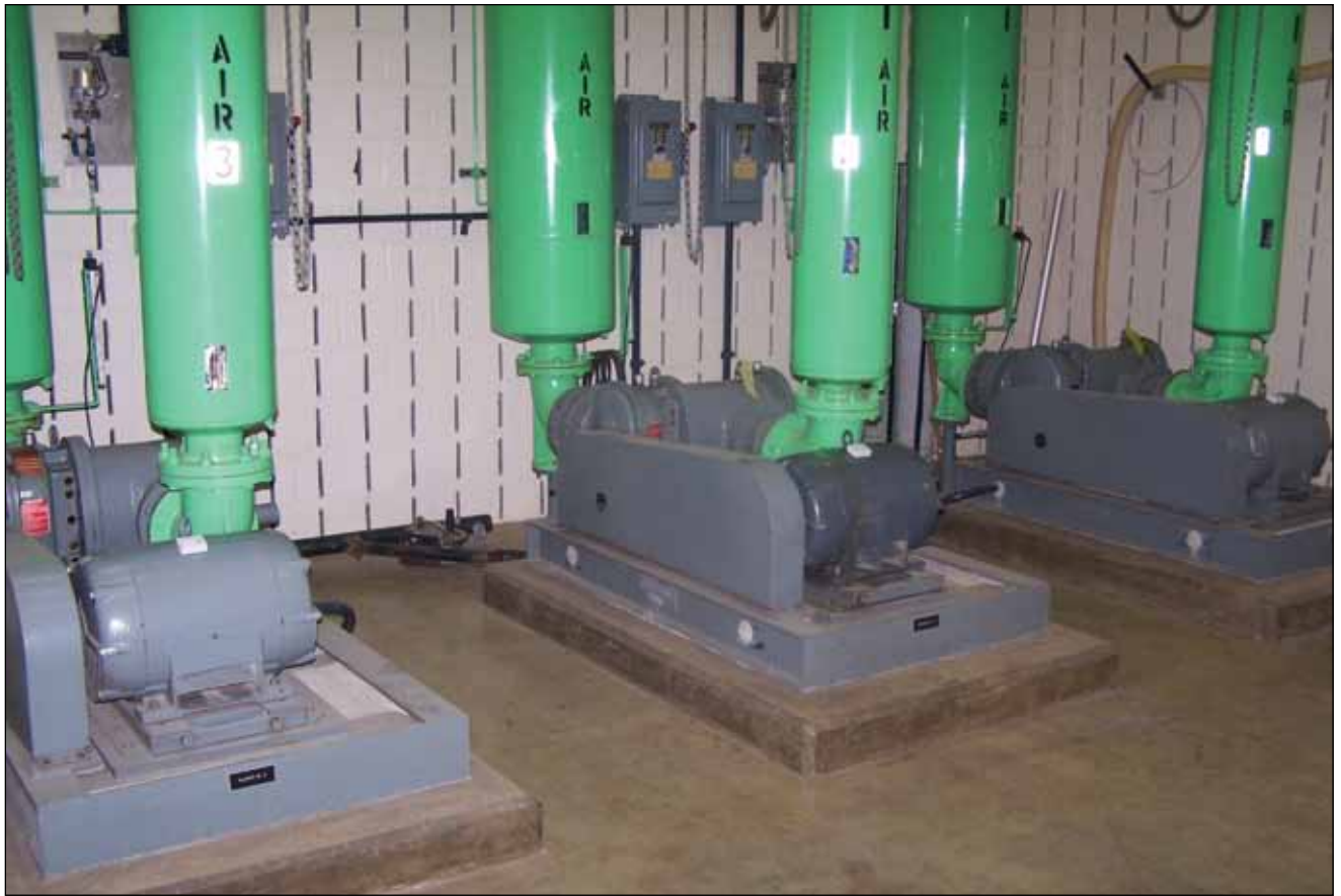
Onset's HOBO U9 Motor On/Off data loggers were attached to the motors to conduct a detailed energy audit. The focus was on the aeration process, which is comprised of motors and fans and is the plant's biggest energy thief.
