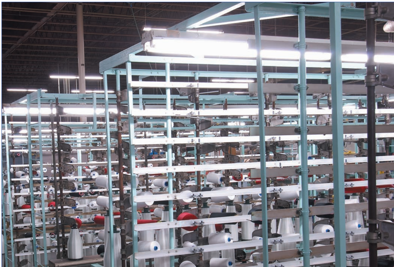
Aerospace supplier ORCON Corp. saved almost $55,000 in energy costs through a lighting retrofit project Lime Energy was enlisted to help with. (Courtesy of Precision Fluorescent.)
