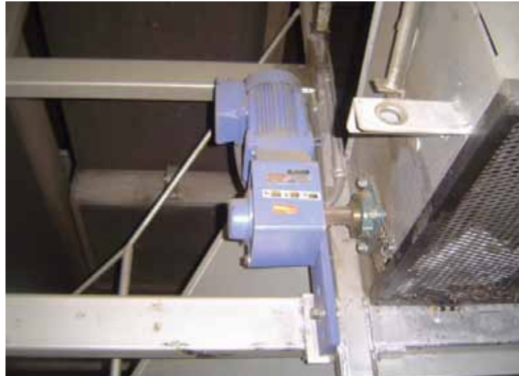
Figure 6—Example of improper installation.
