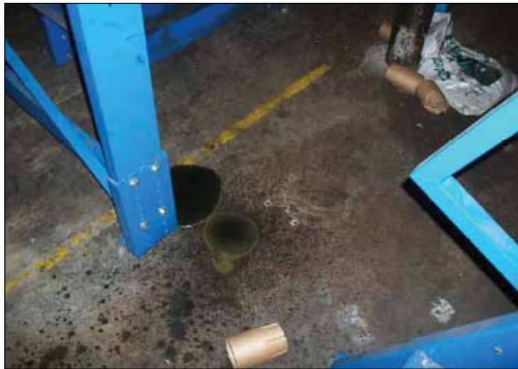
Figure 8—Example of seal failure.
