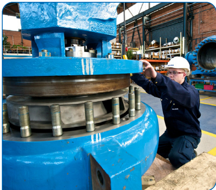
A well-organized pump repair workshop reduces downtime and minimizes costs.
