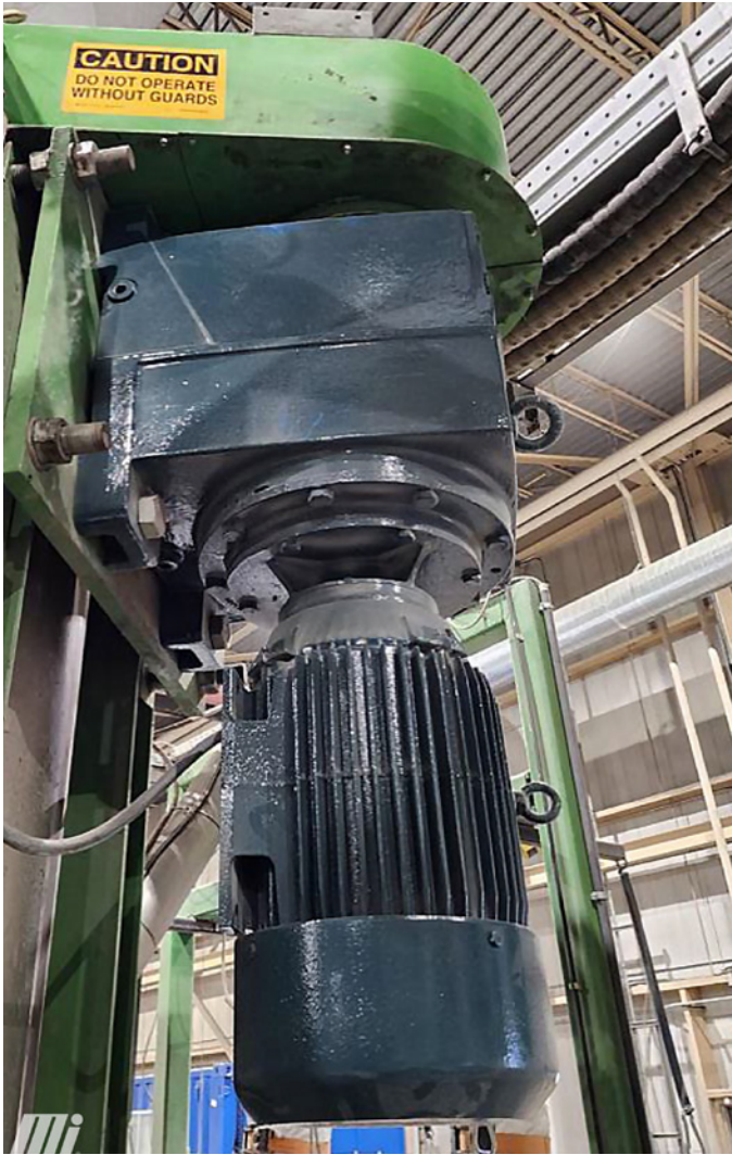
Used in a foam recycling mixer application, this gearmotor features a C-face to protect the motor from the oil and to provide a dry connection between the motor and the gearbox. In case of a motor failure, the facility can swap the motor without touching the gearbox. This unit has a speed output of 15 rpm and a torque output of 115,000 lb.in. Image courtesy of Motion.
