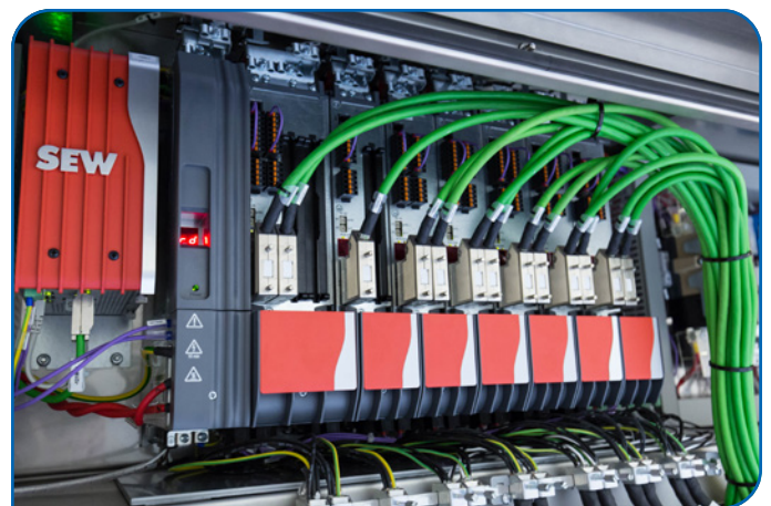
Typical centralized control cabinets house the motor controls, PLC, and circuit protection. Motors and other devices are wired back to this central point. (Image courtesy SEW-Eurodrive)
