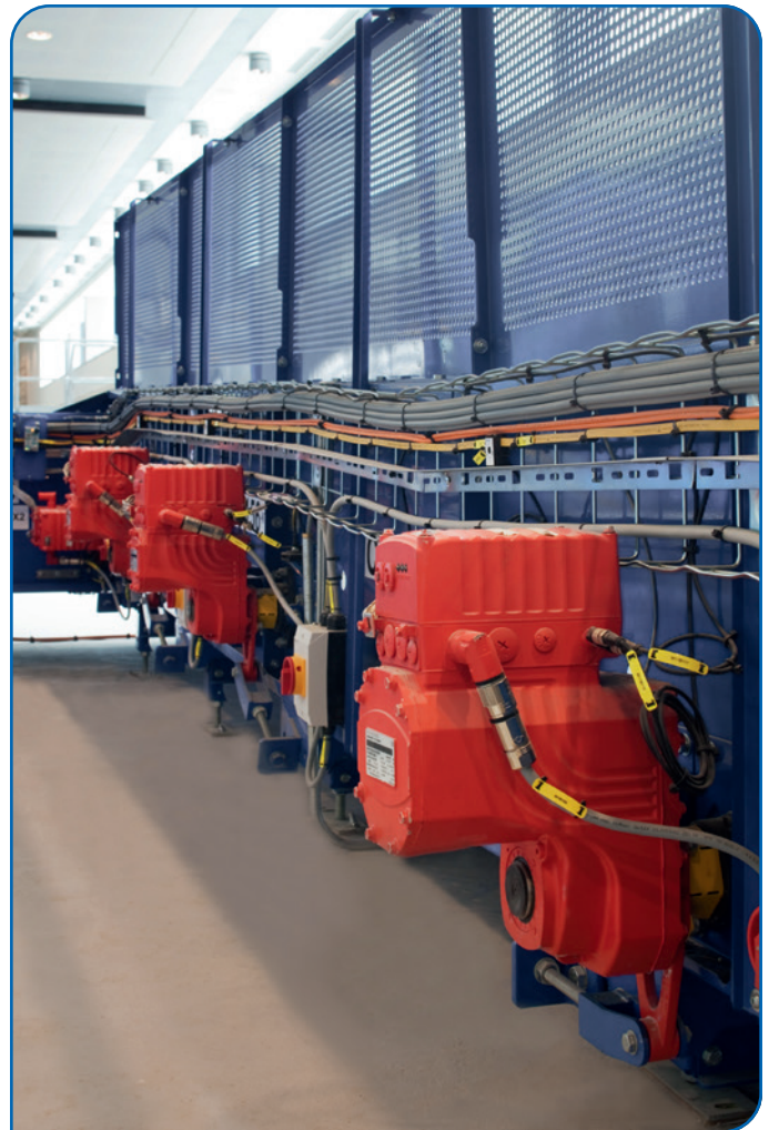
Applications that have long cable runs and multiple axes are typically the best opportunity for a decentralized control installation. Machine expansion can also be easier and less expensive. (Image courtesy SEW-Eurodrive)
