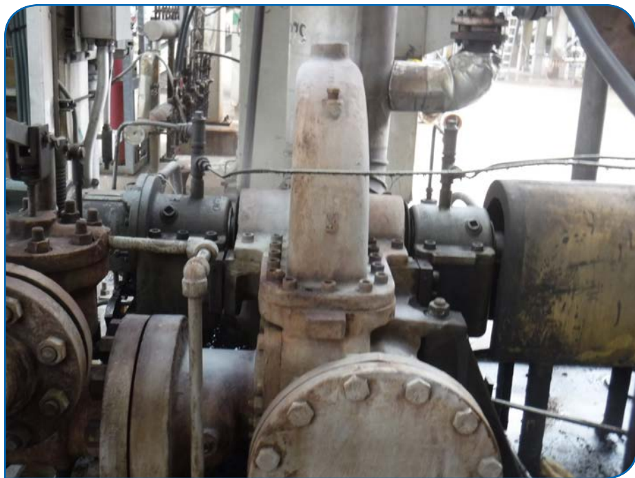
Outdoor boiler feed pump at a refinery in Canada with thermal growth issues due to seasonal pipe strain.
