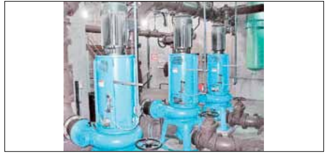
Figure 17—Pump system in a water treatment installation.
