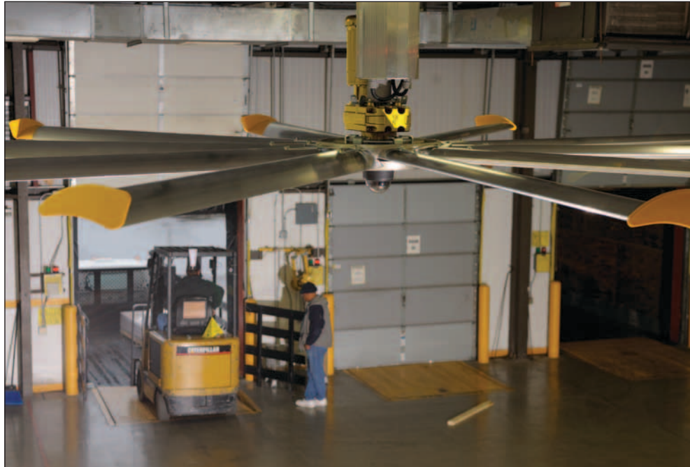
The hollow output shaft creates a stationary platform for integrating electrical functions, like lights, cameras, motion sensors and smoke detectors.
