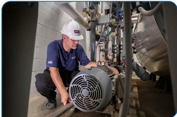
Perceptive Technologies install.
